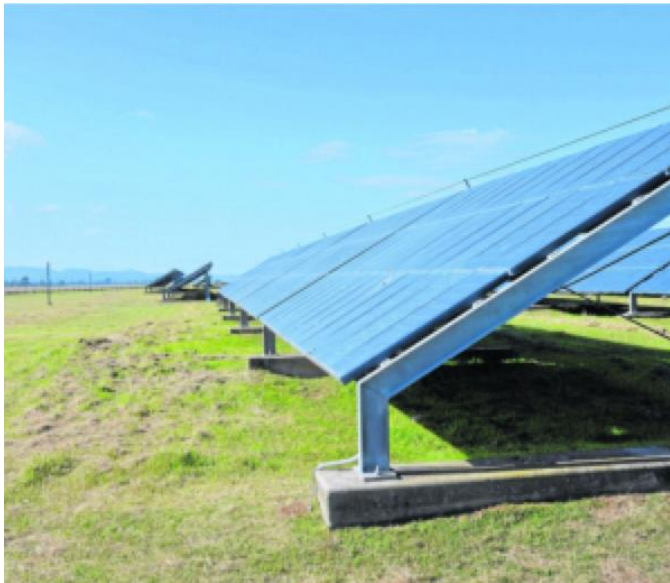
200kW Singleton Solar Farm
