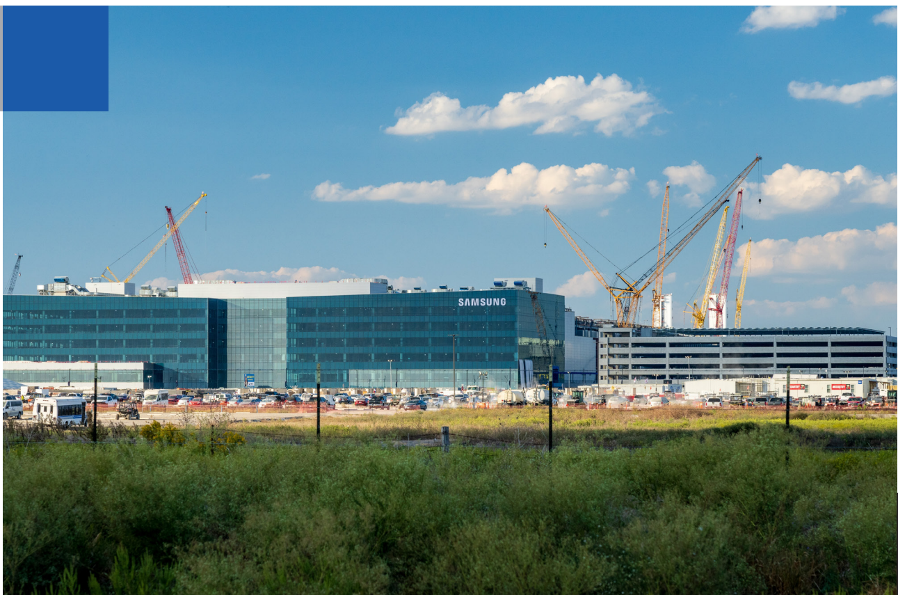
Construction continues on Samsung’s six million square foot manufacturing facility located in Taylor, Texas on October 5 2024 (Steve Heap / Shutterstock)
