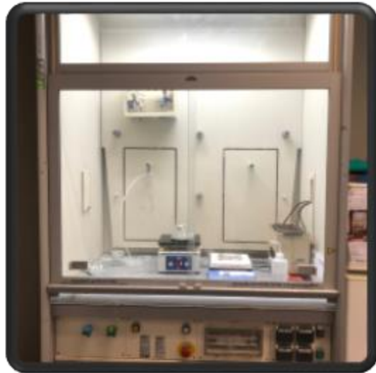
Ducted Fume Hoods
