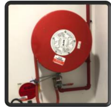
Fire Hose Reel (water)
