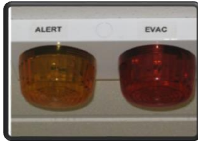
Note ALERT and EVAC flashing lights in corridors and labs for hearing impaired
