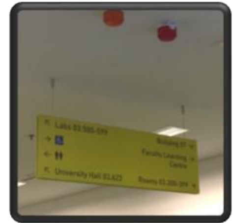
ALERT and EVAC lights in circulation areas
