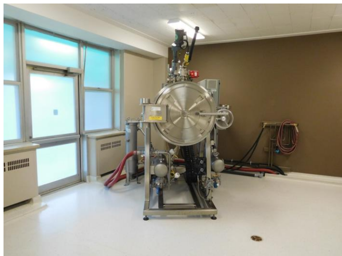
Figure 12: An alkaline hydrolysis facility (source: Bio Response Systems).
