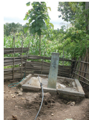
Water system in disrepair
