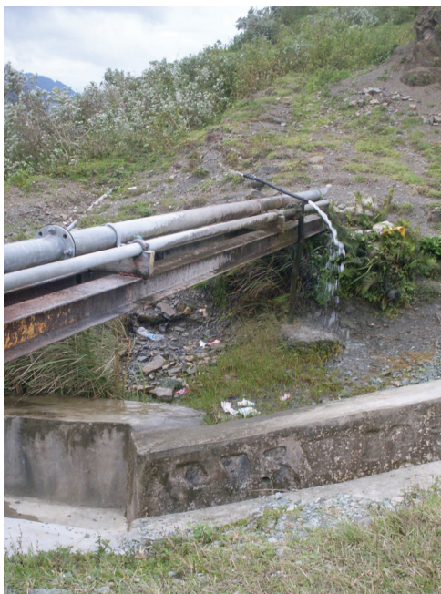
Water system in need of maintenance
