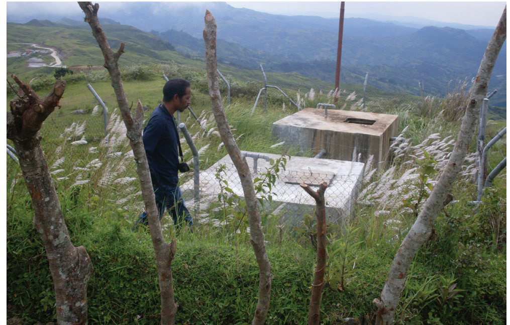
Storage tanks for a gravity-fed water system
