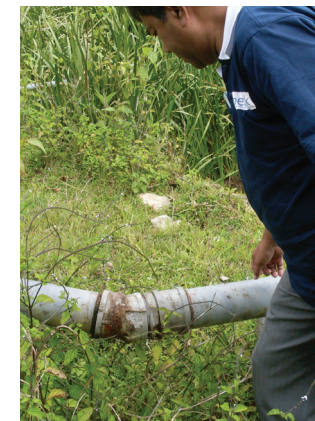
Rusting water pipes
